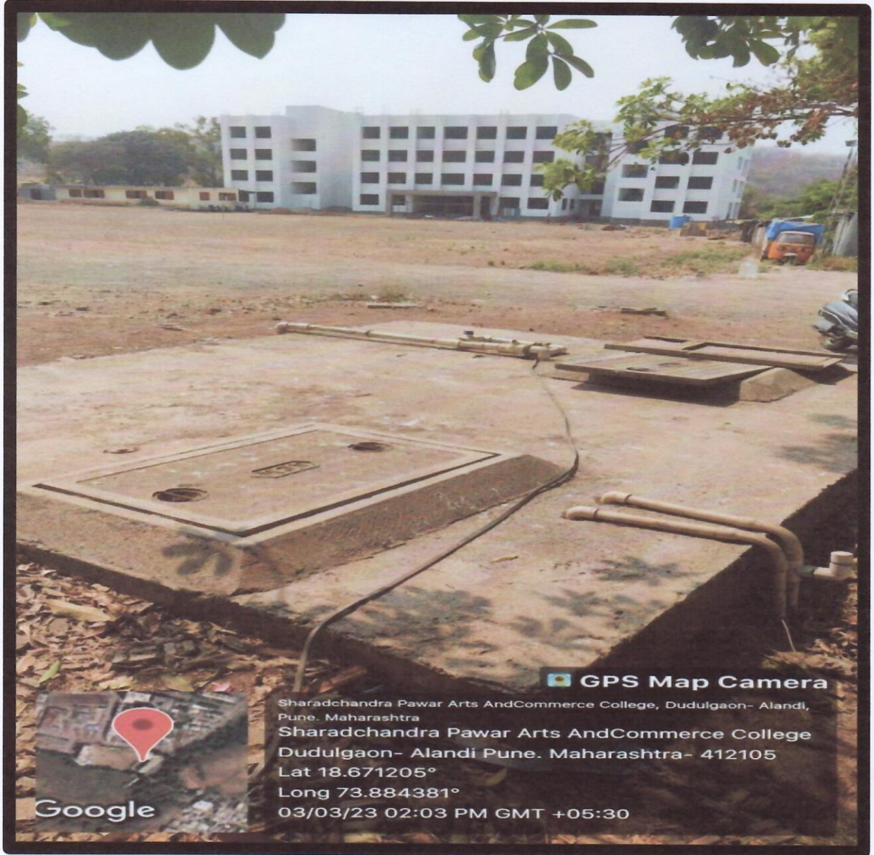
Ground Tank of Water
